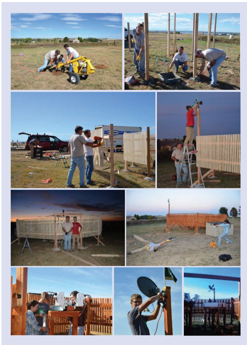
FIGURE 2. The construction of a DFIR double wind fence and the MASC and 2DVD installation at the MASCRAD Easton site (Figure 1) by members of the Electromagnetics Lab at CSU (October 2014). This kind of field construction and instrument installation project, while not entirely sounding like graduate research, and not commonly undertaken directly by university research labs, is an excellent opportunity for students to gain an appreciation of the complexity of real-world research projects as well as some broader engineering skills, advance their rapport among the group and with their graduate advisor, and strengthen the morale of the group and the project team in tackling more conventional, and presumably more difficult, research tasks. Not less importantly, as can be observed from the photos, we had a lot of fun during these sunny October Colorado days and beautiful evenings.
